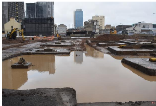
Figure 3.3 Area B and the rear yards of Lots 74 to 76 under water after heavy rain. Photograph taken looking west across the station box excavation area.
